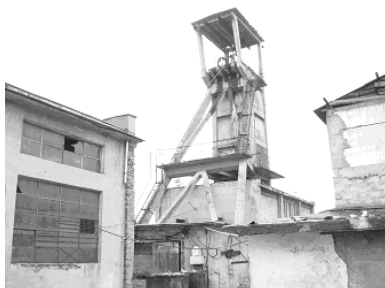
Fig.1. Hoisting device „Auxiliary shaft“
