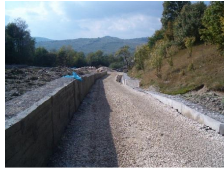
Figure 16 – minor and major riverbeds, rebuilt at the contact between slip and natural slope,
