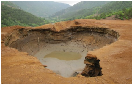
Hole in the dam body
