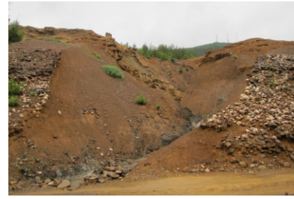
Crack in embankment
